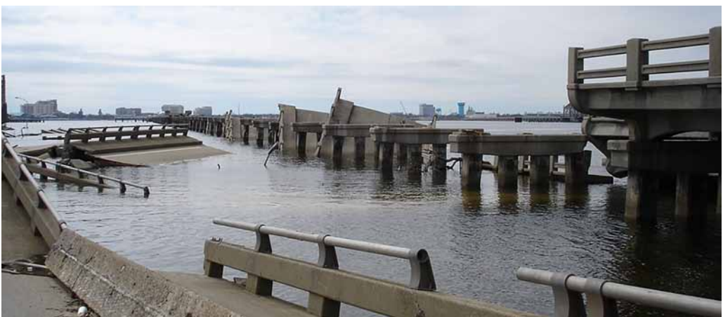
Figure 1.2 Failure of US90 highway bridges east of Biloxi (Courtesy William Allsop)
