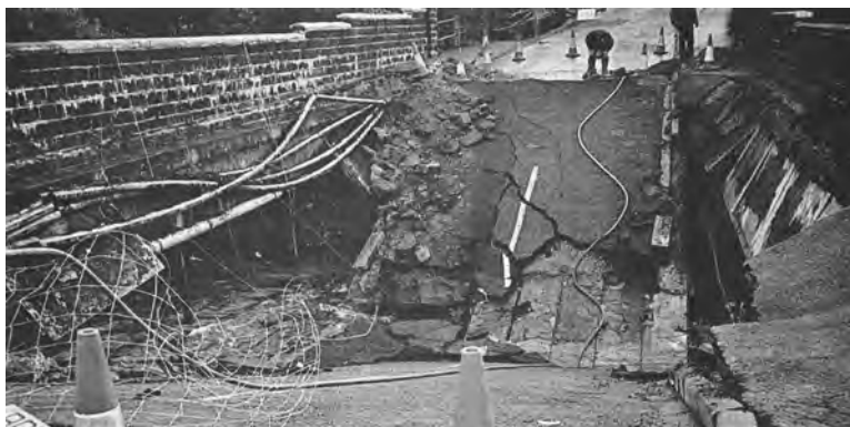
Figure 1.4 The collapse of the Ynys-y-Gwas Bridge led to a ban on grouted tendons [6]
