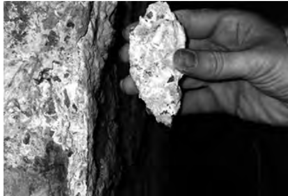
Figure 1.5 Thaumasia attack against a bridge in Gloucestershire
