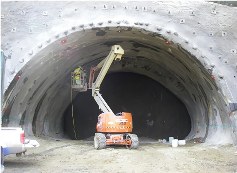
Figure 7.4 Pipe arch canopies installed in a stepped umbrella array (A3 Hindhead Tunnel)
