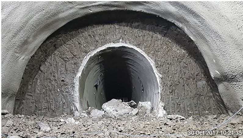
Figure 6.7 SCL pilot tunnel in a top heading invert enlargement (Bank Station Capacity Upgrade)
