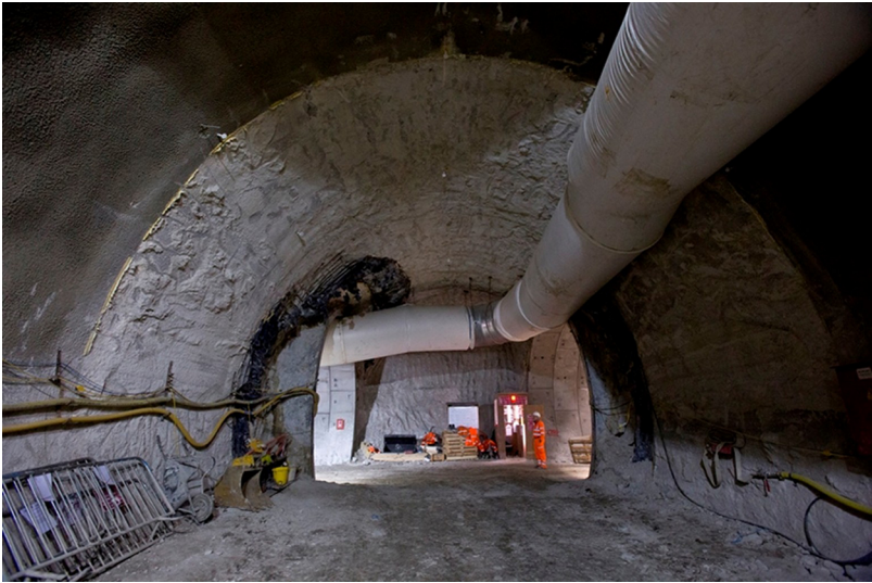
Figure 6.11 Connection into TBM Pilot Tunnel from a backfilled SCL wraparound (Crossrail Tottenham Court Road Station)
