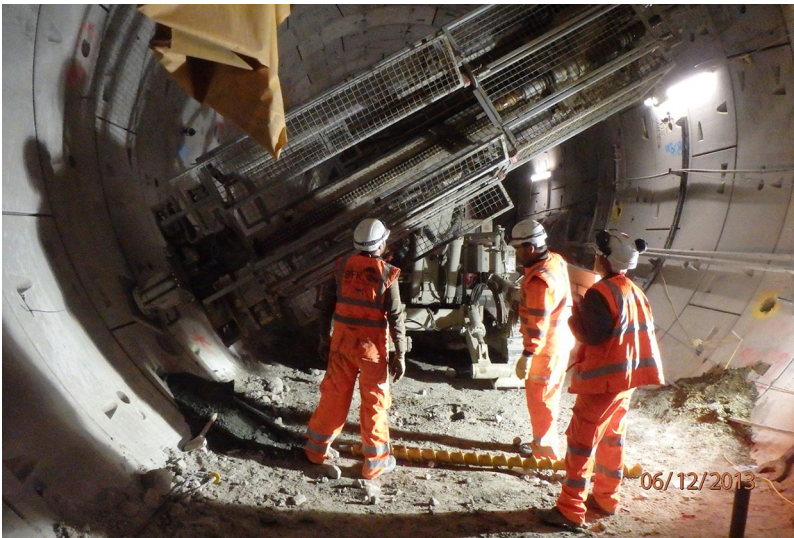
Figure 6.9 Probing from inside a segmental pilot to facilitate an SCL enlargement (Crossrail, Farringdon Station)
