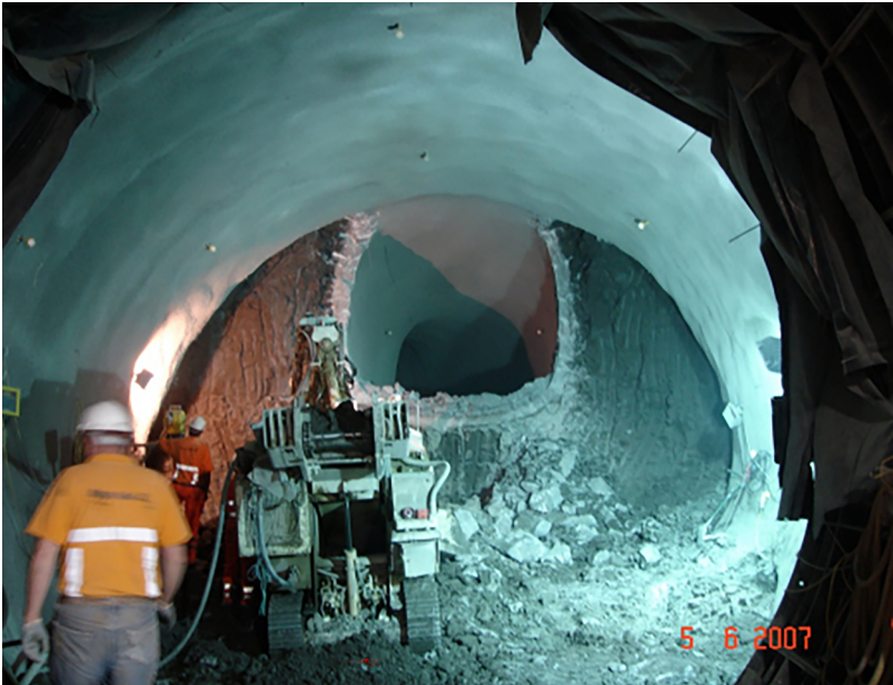
Figure 6.10 Pilot tunnel in the crown of a tunnel (Kings Cross Station upgrade)
