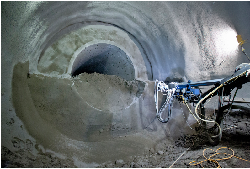
Figure 6.8 Segmental pilot tunnel in a top heading invert enlargement (Crossrail, Tottenham Court Road Station)
