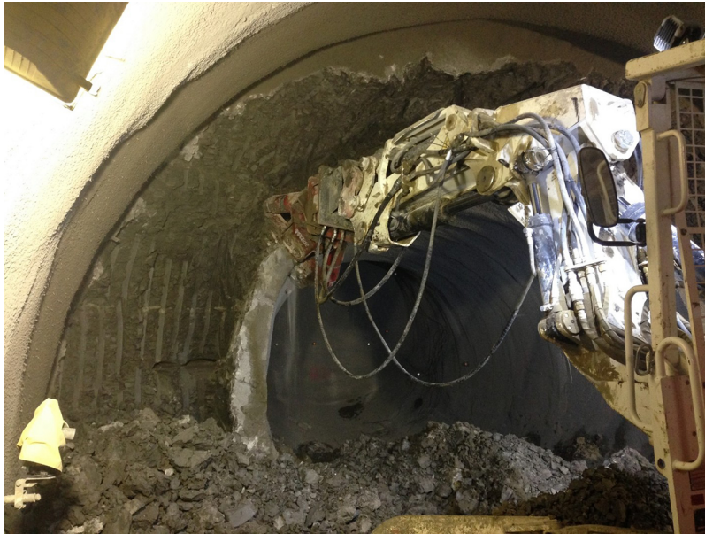
Figure 6.13 Excavator attachment used to break out a pilot tunnel (Bond Street Station Upgrade)
